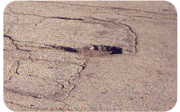
A once smooth road surface has cracks and fractures, plus a large pothole.
